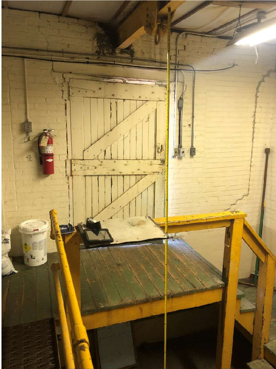
Proposed Structural Steel Vertical Load Support Column – South Column Proposed Location – See Structural Steel Specs – Place W16 x 26 105" from Existing Floating Beam to New Proposed Concrete Pier Placed 60" Above Basement Floor.
