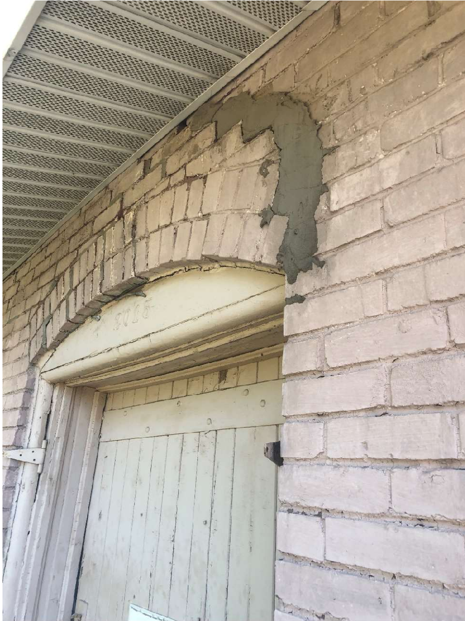
South Elevation, Door Detail View – Active Failure Area Above Door Arch
