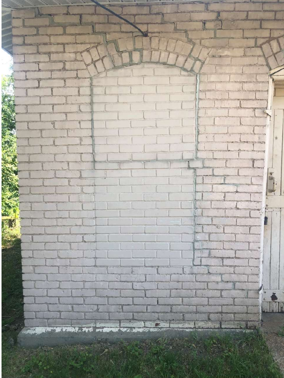
South Elevation, West Window Detail View – Active Failure Area Above Window Arch and Mid Centerline of Window
