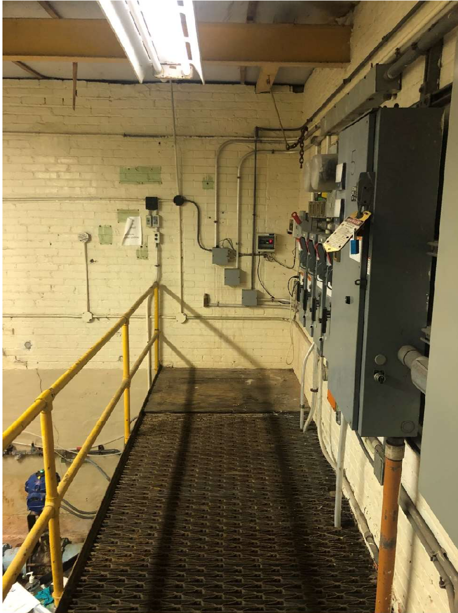
Proposed Structural Steel Vertical Load Support Column – East Column Proposed Location – See Structural Steel Specs – Place W16 x 26 105" from Existing Floating Beam to New Proposed Concrete Pier Placed 60" Above Basement Floor.
