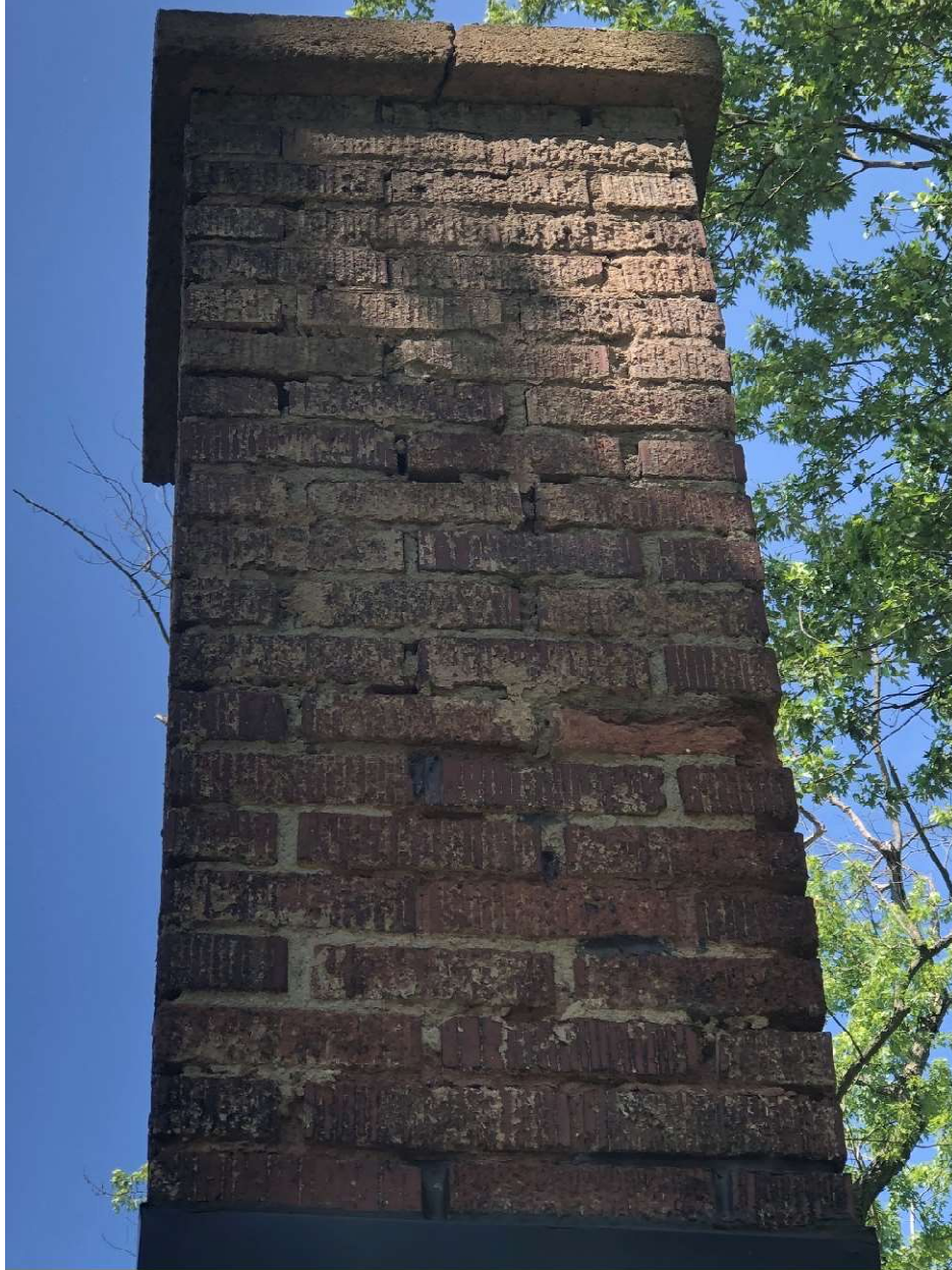
Chimney Detail View – Included Quantity of Masonry Tuck Pointing (Type N Mortar). Concrete Cap Included Quantity of Concrete Restoration (RPS-263 Rapid-Hardening Vertical/Overhead Repair Mortar)
