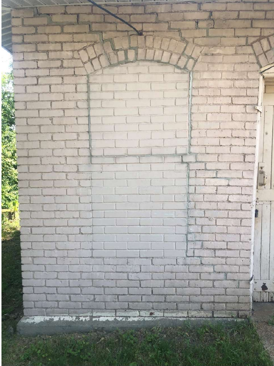
South Elevation, West Window Detail View – Active Failure Area Above Window Arch and Mid Centerline of Window
