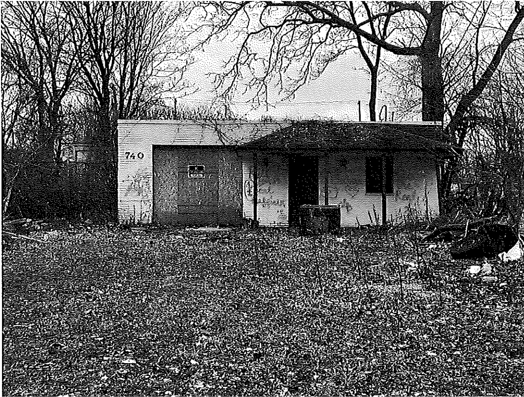
Street view of the building located at 740 E. Vine Street (EA-1) and roof (EA-5)
