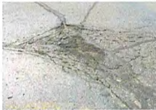
Patch work needed
