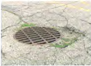
Drain needs repairing
