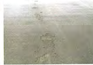
Traffic topping damage
