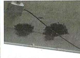
Leak in ceiling
