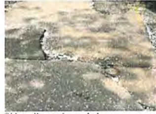
Sidewalk repair needed
