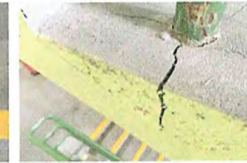
Crack in stairs
