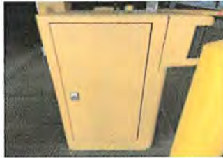
Equipment needs painting
