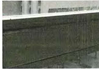
Rusting on South Street
