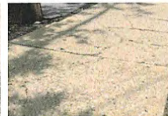
Sidewalk in need of repair
