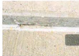
Caulking needed rooftop
