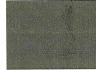
Farmers Alley wall crack
