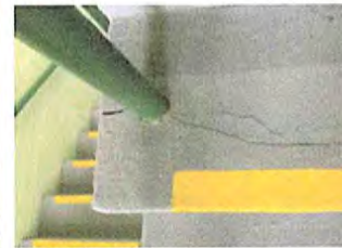
Crack in stairs
