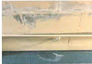
Moisture problem back hallway
