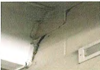
Crack in brick wall
