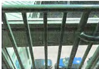
South St. rusting
