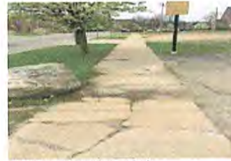
Sidewalk repair needed
