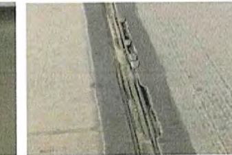
Joint repair needed
