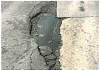
Hole in asphalt
