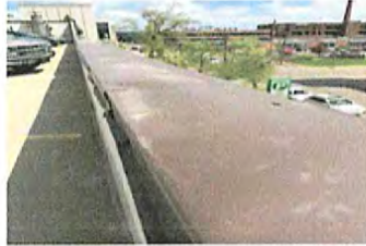
Ledge needs repair
