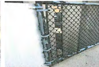
Fence in need of repair
