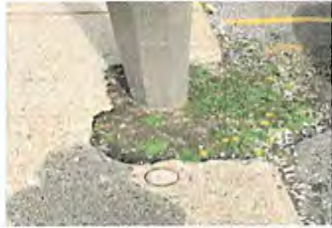
Sidewalk repair needed
