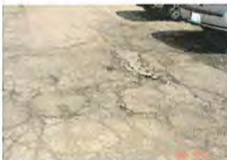
Potholes throughout lot
