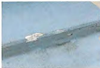
Traffic topping damage
