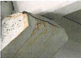
Crack in column
