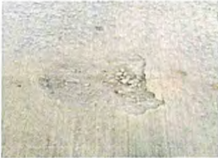
Gouge in concrete
