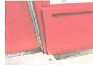
Minor damage to booth
