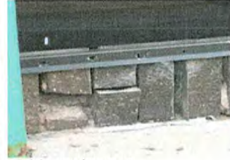
Bricks coming apart
