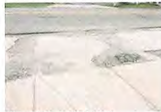
Concrete in need of repair
