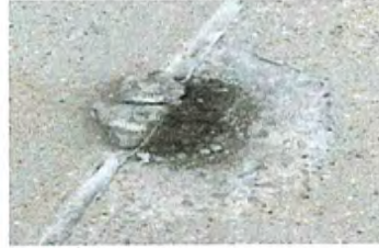
Gouge in concrete
