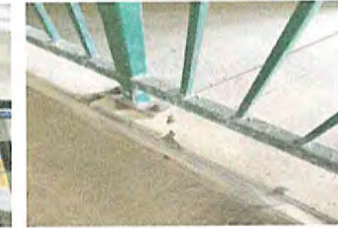
Rusting and need paint
