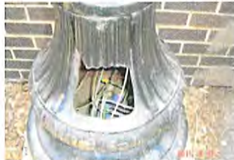
Cover needs to be replaced
