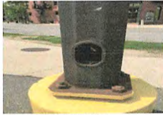
Missing electrical covers
