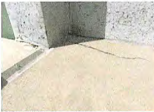
Crack in beam
