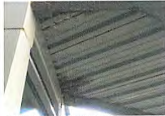
Rusting under crosswalk
