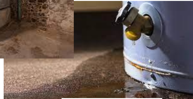
Critical repair Code Repair Homeowner EDU
