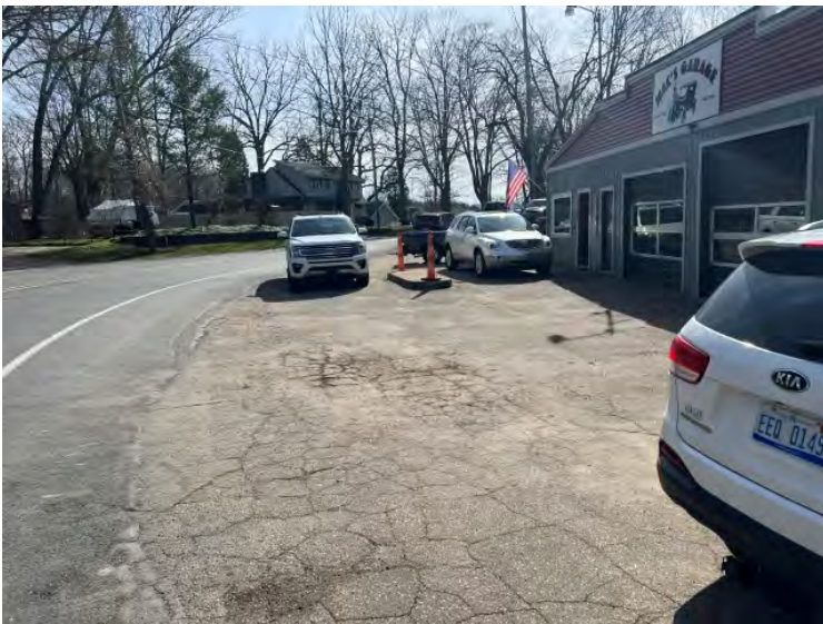
View of a pump dispenser island at Mac's Garage.
