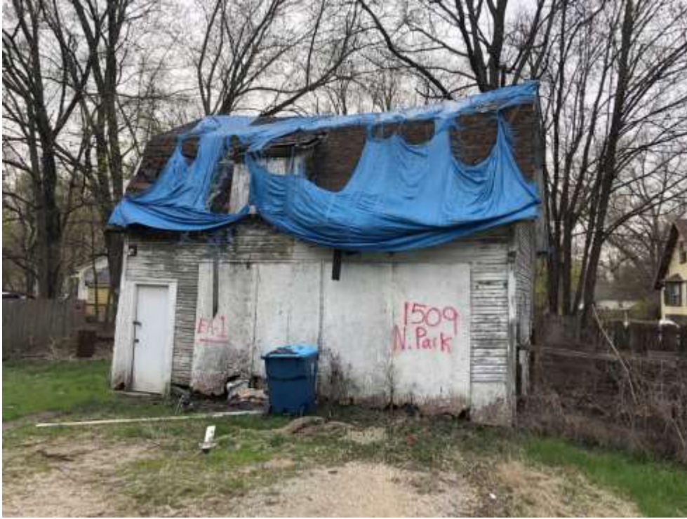
View of the garage located at 1509 N. Park Street (EA-1) and roof (EA-5)
