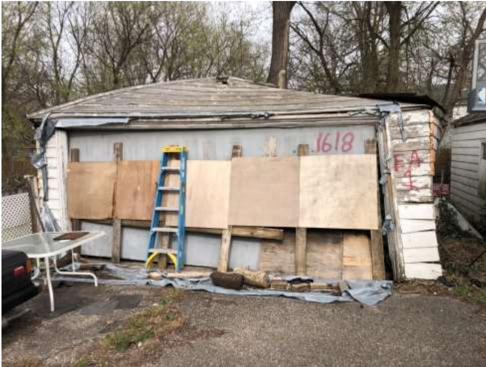
View of the garage located at 1618 N. Park Street (EA-1) and roof (EA-5)
