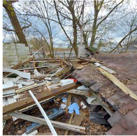
Collapsed Section of Structure (Looking North)
