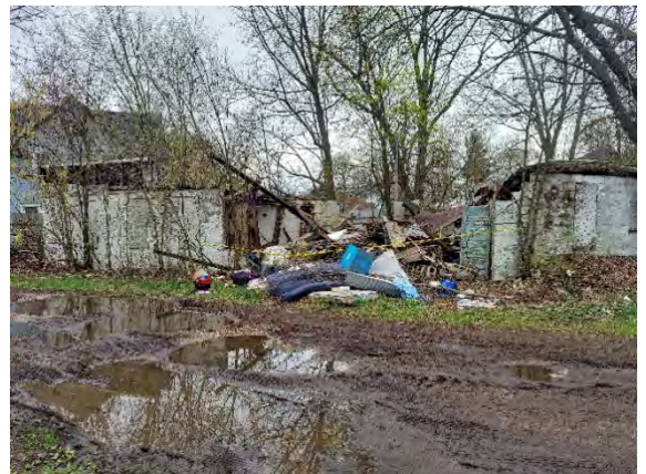
*Due to collapsed structures, additional ACM may be present on the interior of the foundation.
