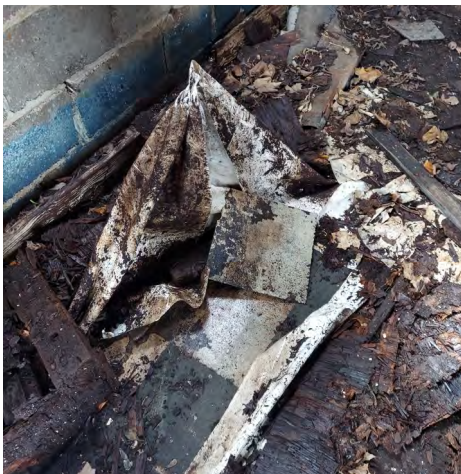
Tan 12x12 Floor Tile, Room 1
