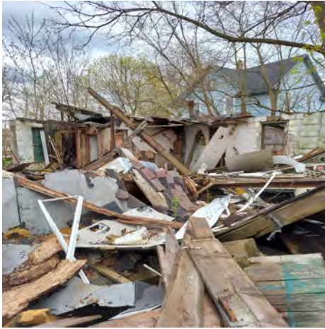
Collapsed Section of Structure (Looking South)
