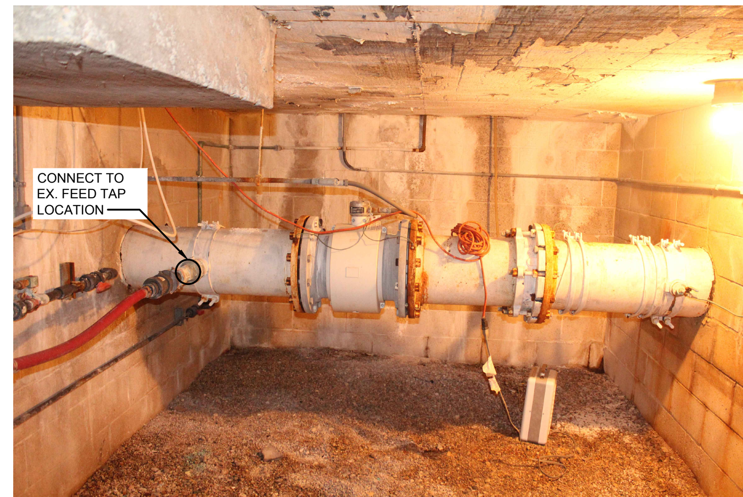
PHOTO 12-1 - FEED TAP LOCATION (BASEMENT)
