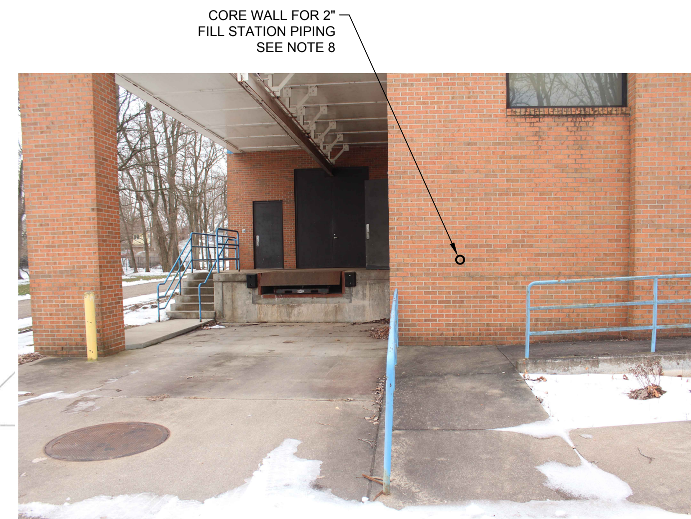
PHOTO 1-3 - PHOSPHATE FILL STATION
