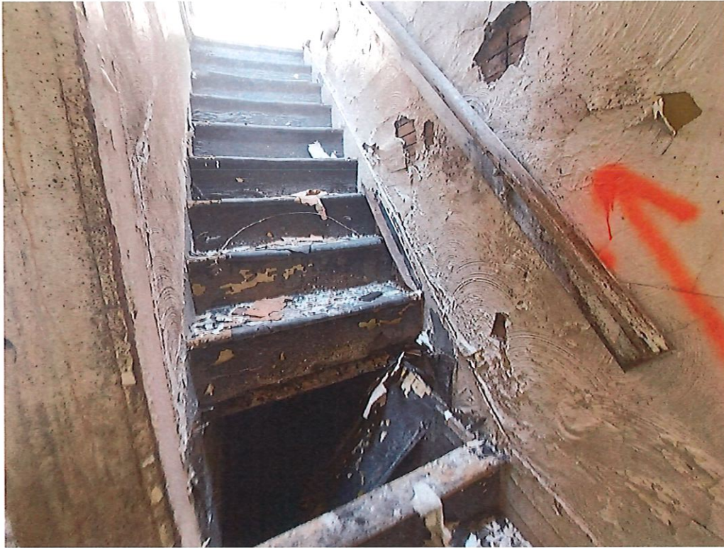
View of FS-11 (Stairs leading to 2 nd floor have collapsed into the basement)
