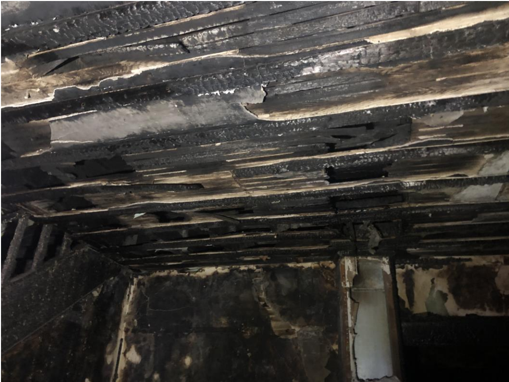
View of the fire damaged 2 nd floor joists continued
