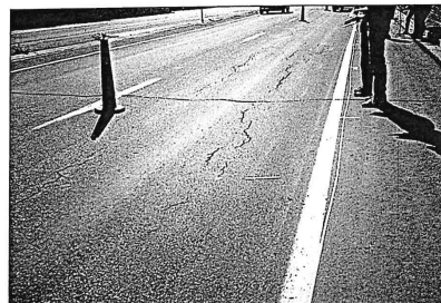
Figure 5: Distress Type ACP 1 - Low Severity Fatigue Cracking
