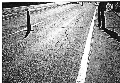
Figure 5: Distress Type ACP 1 - Low Severity Fatigue Cracking
