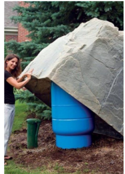
Place Mock Rock Over 8" DIP and 2" HDPE to Conceal Autoflusher Discharge https://allmockrocks.com/ *Minimize Mock Rock Size to Maximum Extent*
