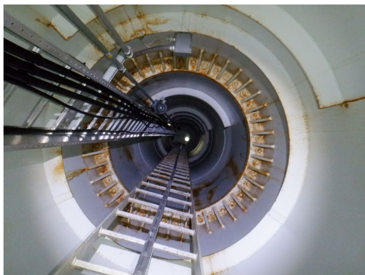
45) The access tube ladder is in good condition. The ladder is equipped with a fall prevention device.
