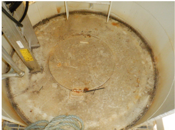
41) Rust bleedthrough on the access tube floor.
