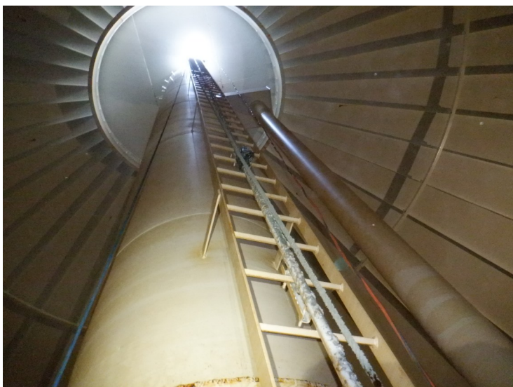
57) The wet interior ladder is in good condition. The ladder is equipped with a fall prevention device that is covered with mineral deposits.
