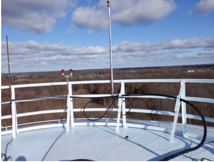
19) The roof handrail is in good condition. The handrail is being used for antenna mounting.
