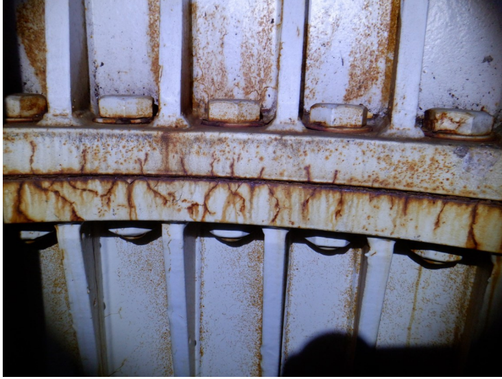
43) Rust bleedthrough at an access tube bolted connection.
