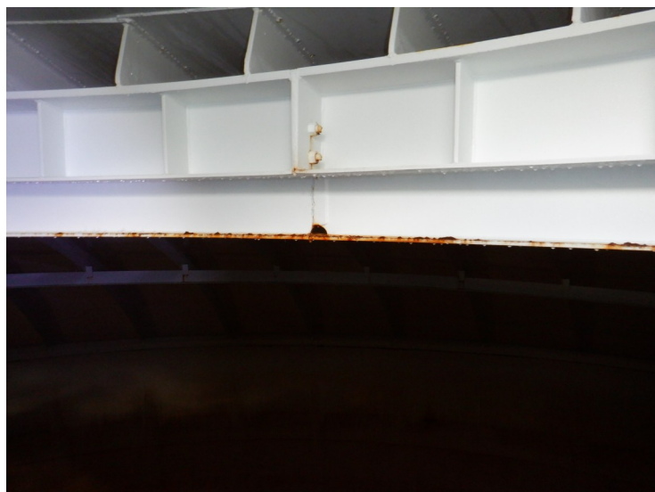
48) Minor corrosion on the roof stiffeners.
