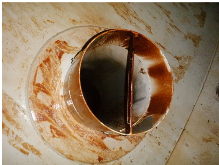
66) The fill/draw pipe is in good condition. There is a deflector bar on the pipe.
