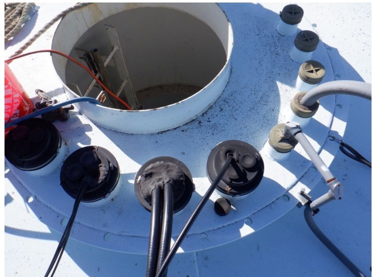
14) The cable routing penetrations through the access tube cover plate are sealed with rubber boots that are in good condition.
