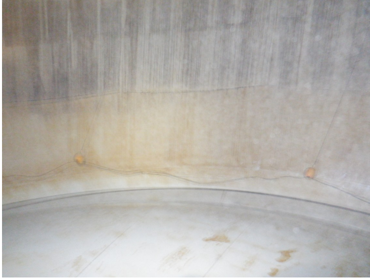
58) The floating ring cathodic protection system appears to be in good condition.
