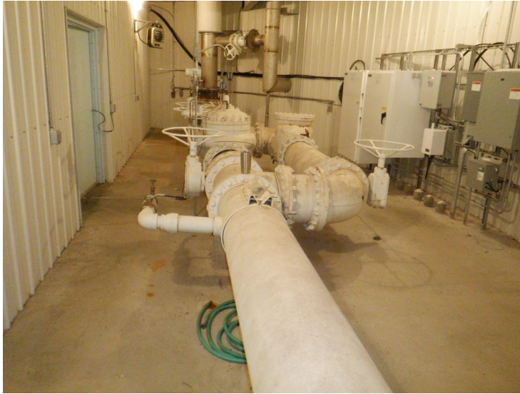
28) The tank piping is above grade in a heated room in the column.
