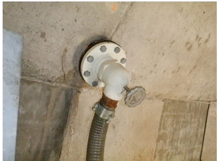
38) The mud valve was not operated during the inspection.
