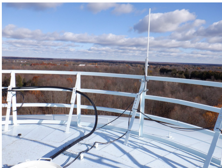
18) The roof handrail is in good condition. The handrail is being used for antenna mounting.
