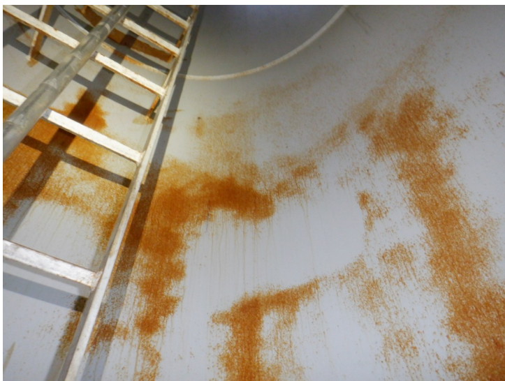
42) Rust bleedthrough in the access tube.
