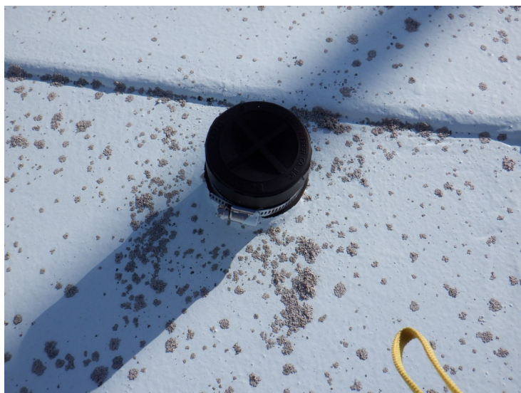
21) Typical roof rigging coupling sealed with a rubber boot.
