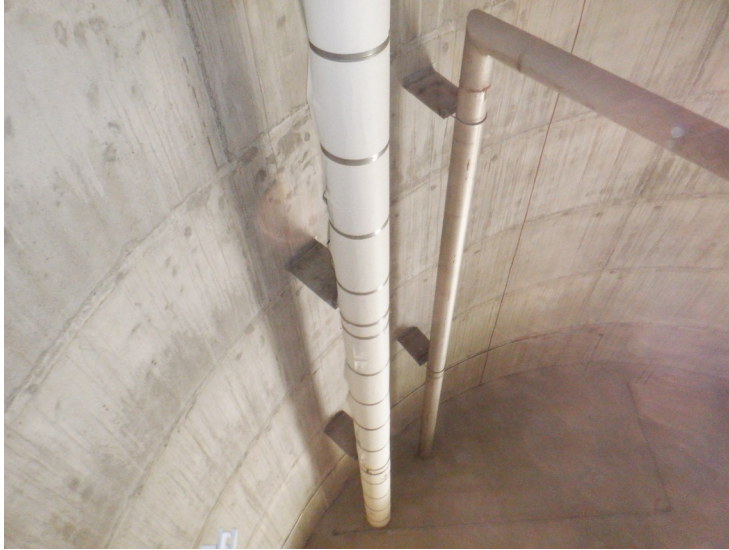
37) The fill/draw pipe insulation is in good condition. The paper cover is loose in a few areas.
