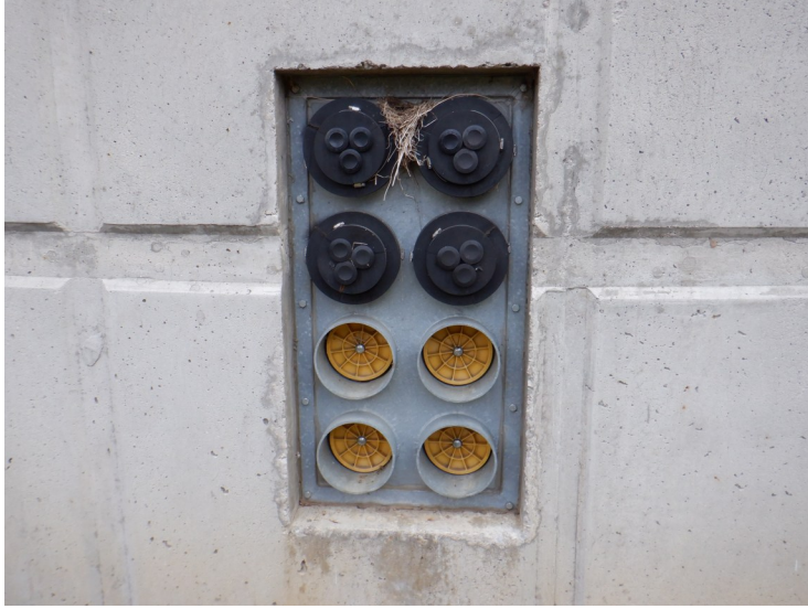
4) The antenna penetrations in the bottom of the column are sealed with rubber boots and plastic plugs that are in good condition.
