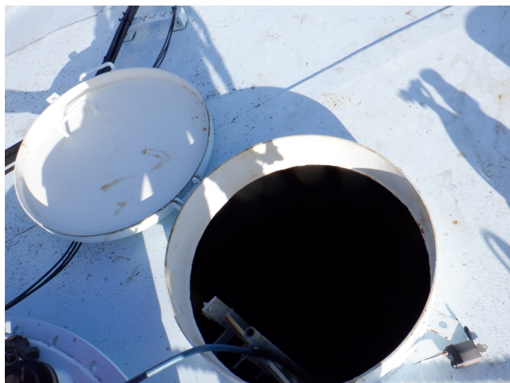
27) The wet interior roof hatch is in good condition. There was no gasket on the hatch.
