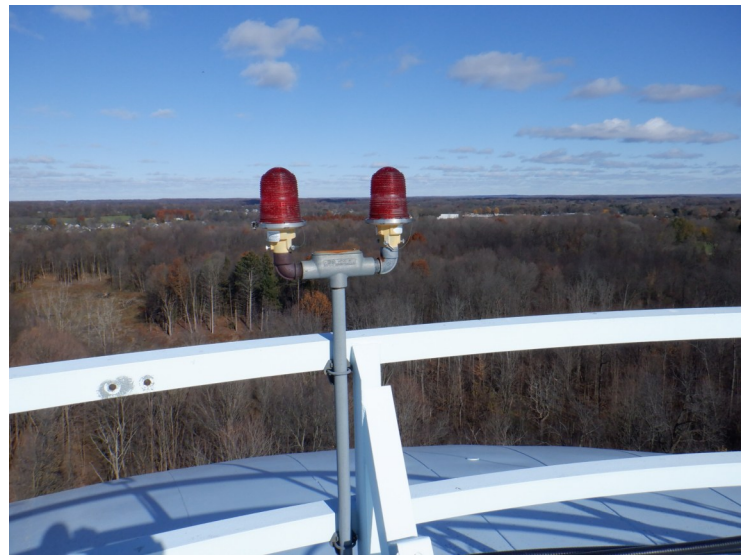
20) The double red aviation light appears to be in good condition but it is unknown if it is functional.
