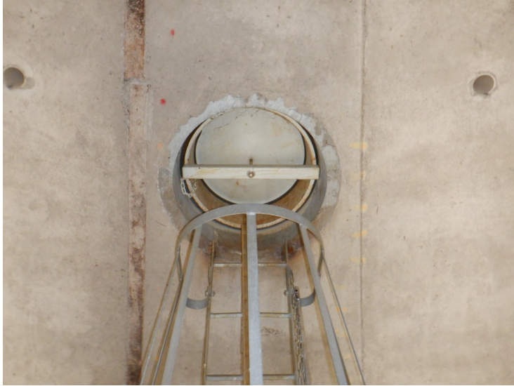
40) The manway to the wet interior in the domed bottom is in good condition.
