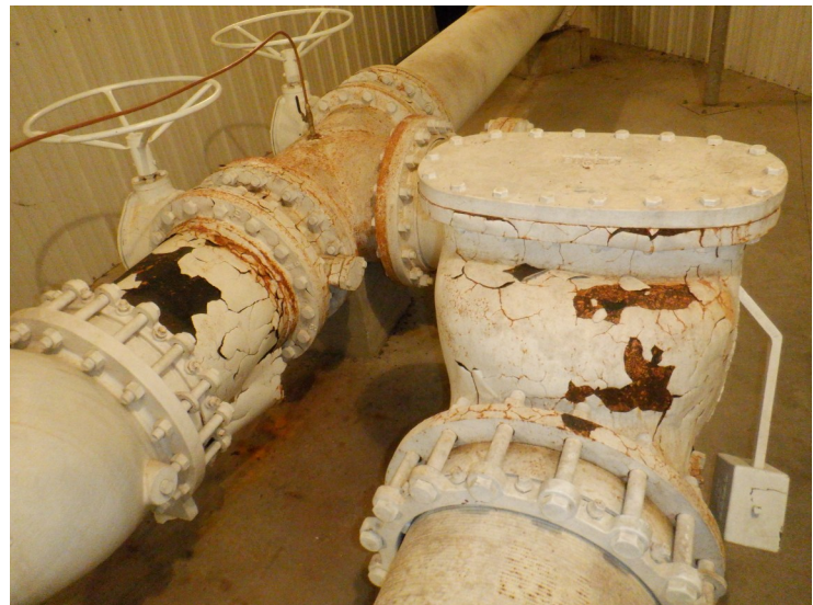
29) The pipe coating is in poor condition overall.
