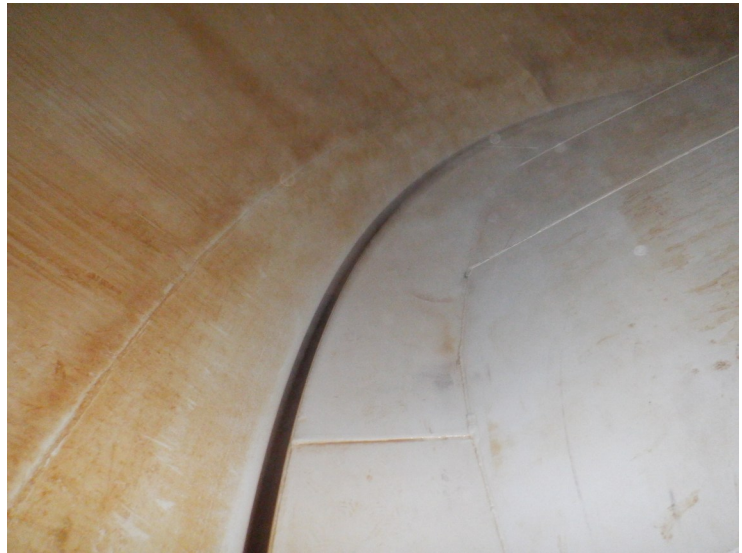
62) The bottom bowl coating is in good condition.
