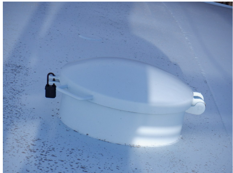
23) The two secondary wet interior roof hatches outside the roof handrail are in good condition.
