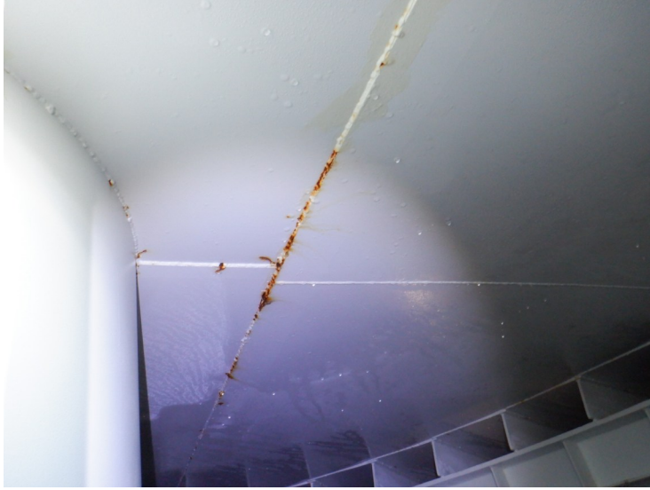
46) Spot coating failures on the wet interior roof at the weld seams.
