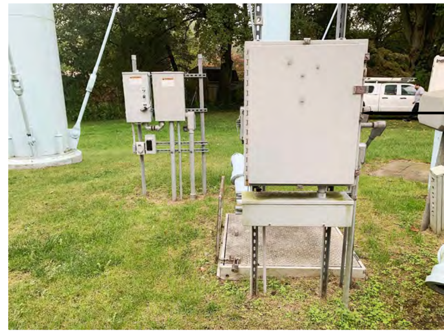
EXISTING PLC PANEL
