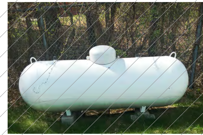
SAMPLE PROPANE TANK
