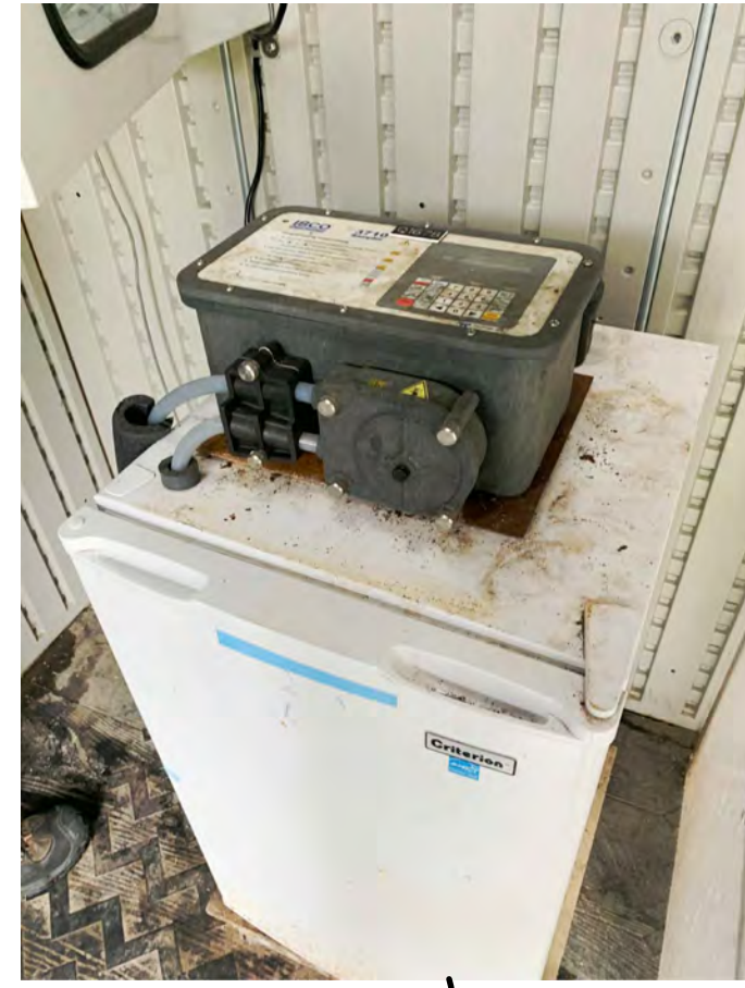
METERING CONTROL PANEL 1" C(2/C#16SH)
